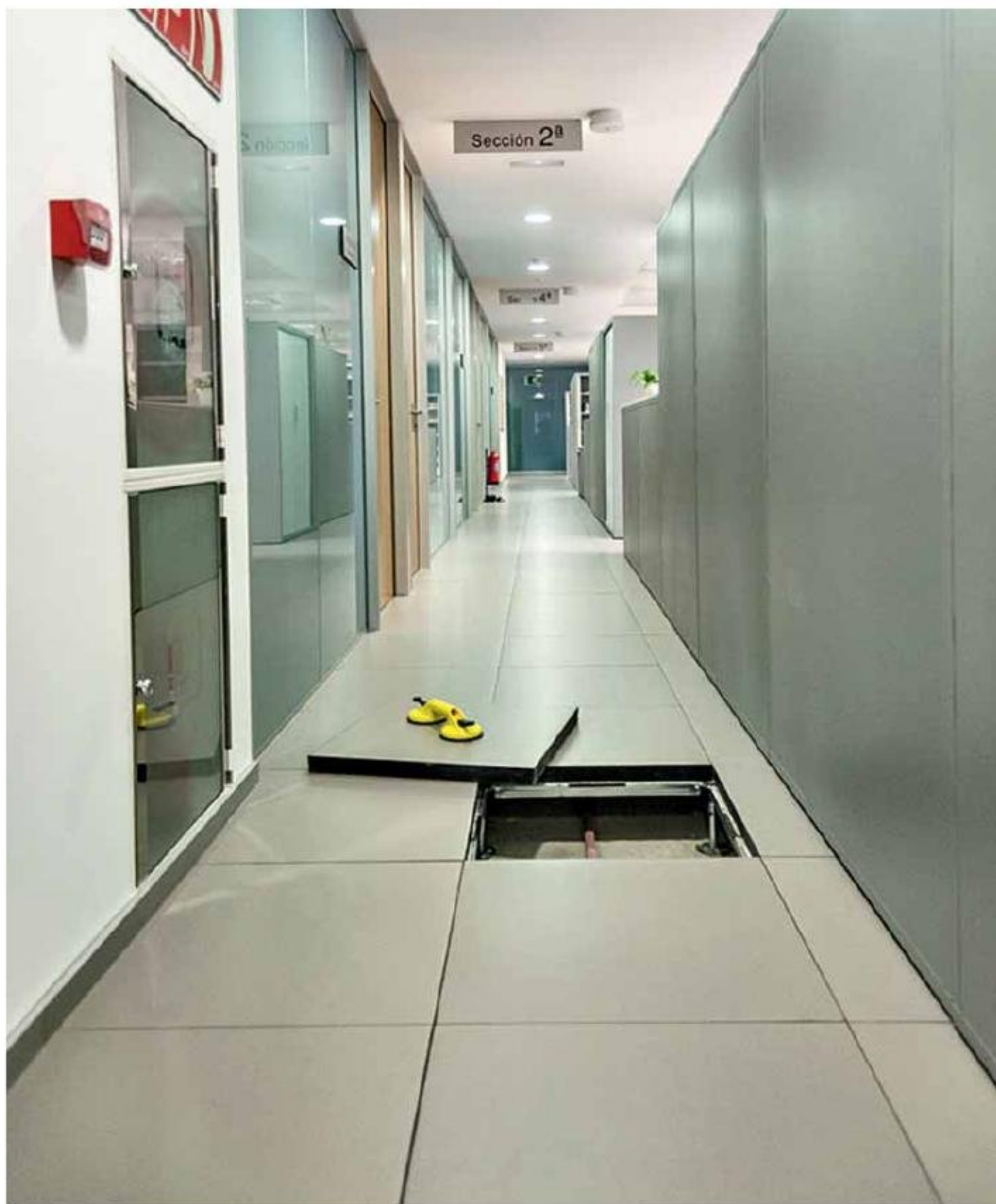
Access floor in the Zaragoza Provincial Courts facility. Porcelain stoneware by Pamesa Cerámica, Cosmos series.
